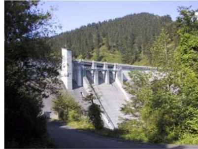
In the case of dam projects, the analysis of hydrogeological characteristics and the
