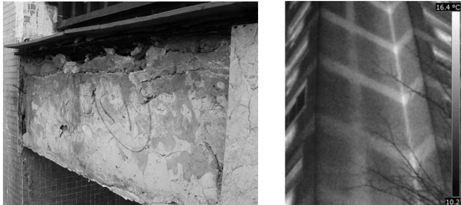
Figure 47 Image of a constructive problematic points of the current building and thermal bridges of front of slabs and integrated pillars in the facade. Source: Retegui & Altuna and Aurea Consulting
