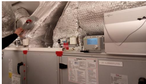
Figure 3: The ventilation unit
