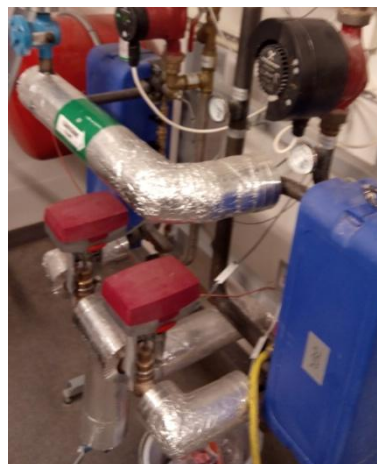
Figure 2: The heat exchangers
