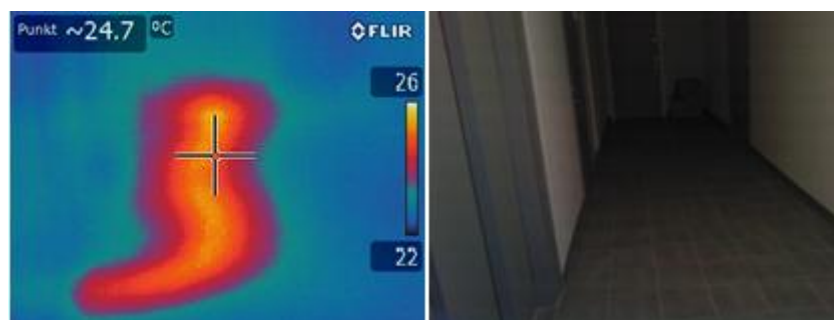
Figure 18: A badly insulated pipe
