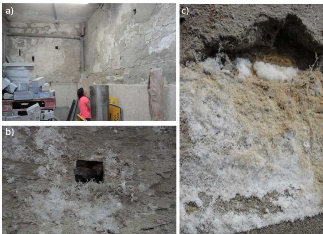
Figure 6.7. Selected photographs of the affection observed in the masonry wall of the groundfloor. a) Salt efflorescence and detachment of the plaster of the wall. b) Accentuated precipitation of salts around putlog holes. c) Enlargement of one of the most affected areas in which the efflorescences, the layer of Portland cement plaster and the original sandstone masonry can be observed.
