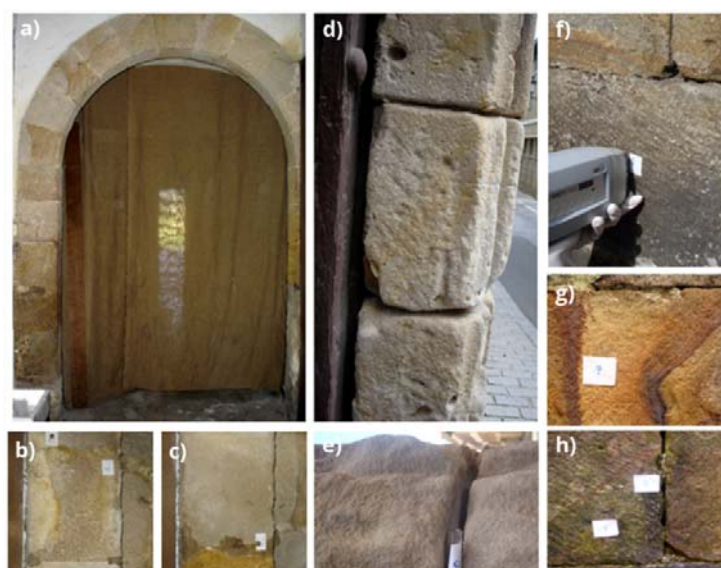
Figure 5.3. Selected photographs of the affections observed in the Palace. a) general view of the central wall arch. b-c) details of efflorescences found in the arch. d-e) material loss observed in the ashlar of the main entrance. f) example of in situ analysis of blackened areas. g) areas with change of coloration. h) biodeterioration and efflorescences found close to the drainpipe.
