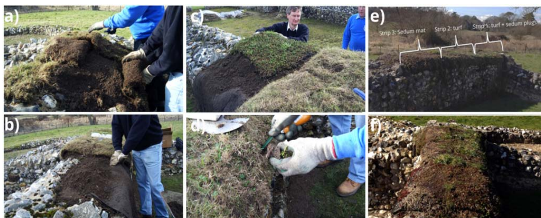
Figure 7.8. Establishment of soft caps. a) Placing the turf layer .b)Securing the sedum mat. c) Management the blocks. d) Adding the sedum plugs. e) The Soft capping test areas finished. f) Top of the test areas (viewed from East).
