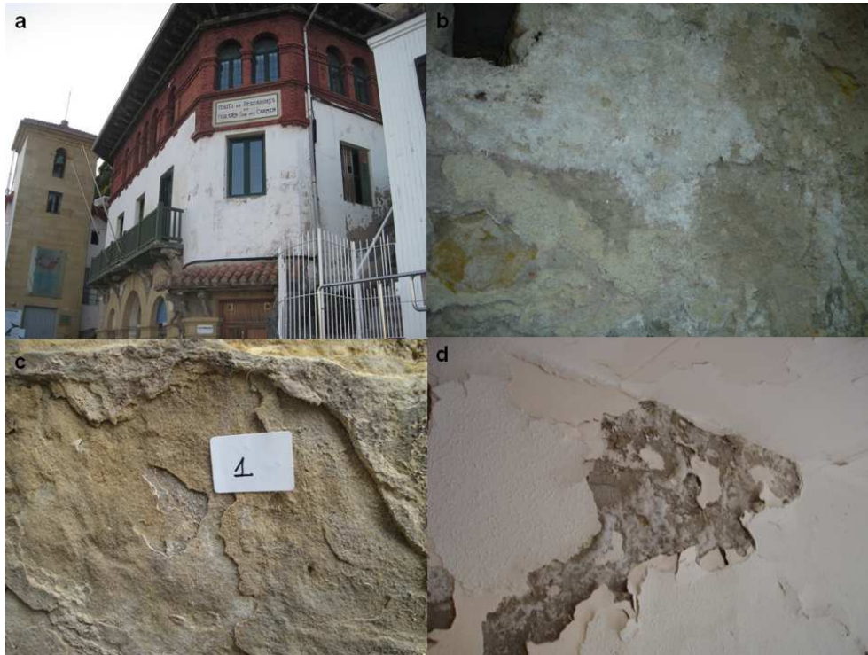
Figure 8. a) Fishermen's association building (San Sebastian, Basque Country, North of Spain), b) efflorescence salts found in the adjacent hill wall of the ground floor, c) flaking and alveolization process suffered by the sandstone of the façade and d) fractures created by the salts migration inside the wall.
