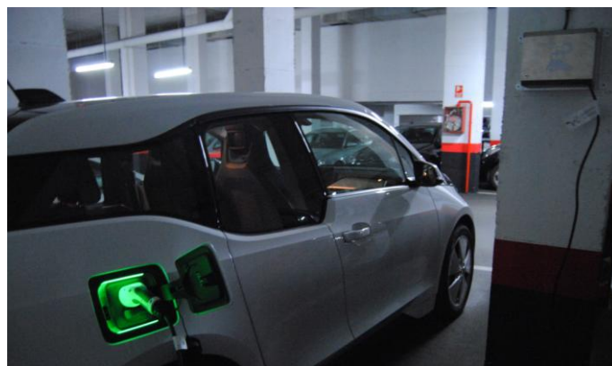
Figure 2.7 Charging point in a community garage.
