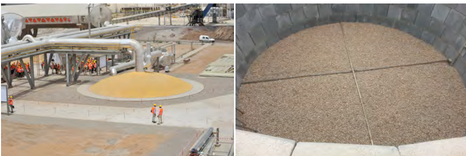
Figure 1.13. Thermocline TES unit constructed by Airlight Energy [125].
