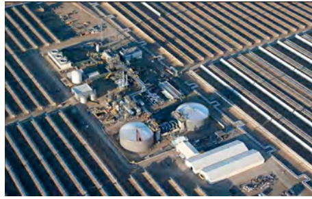
Figure 1.8. Double-tank TES system in the CSP plant of Andasol I [29].
