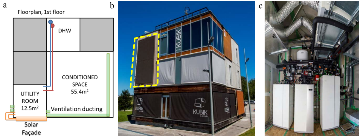
Fig. 3. (a) Floor plan of the Kubik building with the area for tests; (b) South façade of the Kubik building highlighting the solar façade; (c) Utility room with installed equipment.
