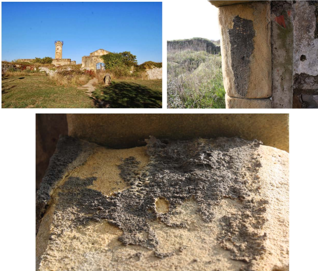
Figure 1.3. Black crusts growing over the building materials of La Galea fortress, a building of the 18 th century (Getxo, Basque Country, Spain).
