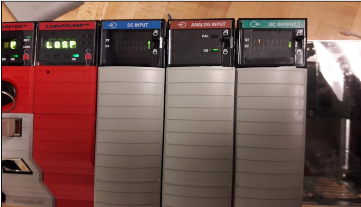
Figure 10: PLC showing output from test routine
