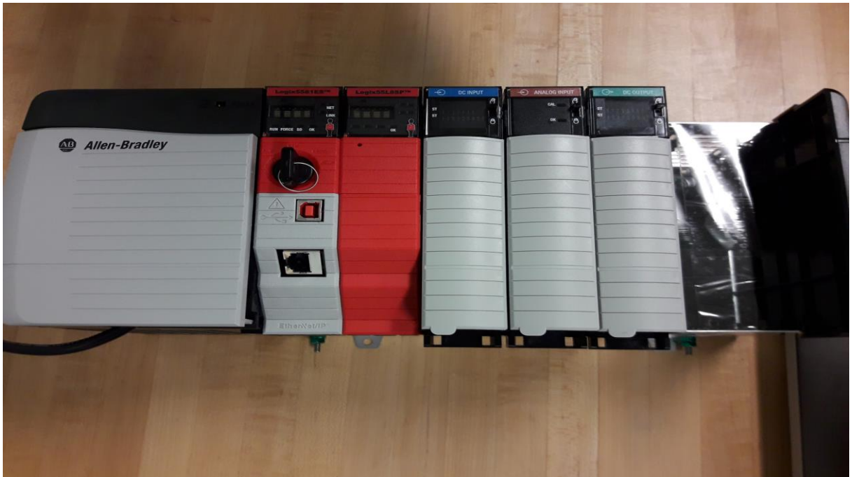
Figure 1: Allen-Bradley ControlLogix 1756-L81ES PLC
