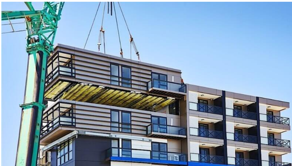
Figure 1.1.1 Craning of a modular unit during the final assembly of the building .
