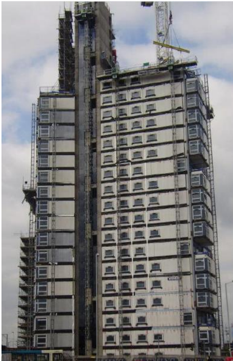
Figure 7.2.2 Photo of the building during its construction, without the exterior finishes. A slab can be seen on each floor, that is connected to the core.
