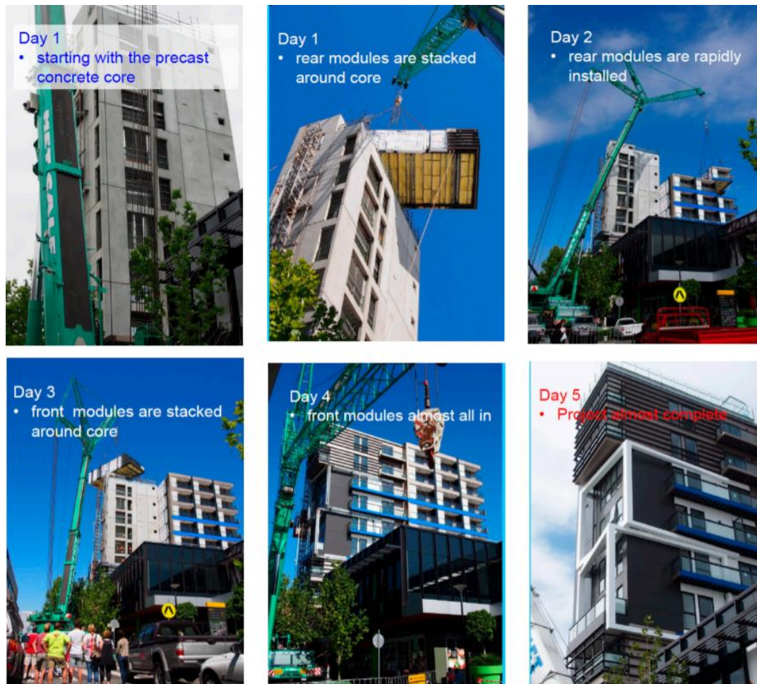
Figure 7.3.1 Performance of Modular Prefabricated Architecture: Case Study-Based Review and Future Pathways (Fred Edmond Boaf 1 , Jin-Hee Kim 2 and Jun-Tae Kim, 2016)
