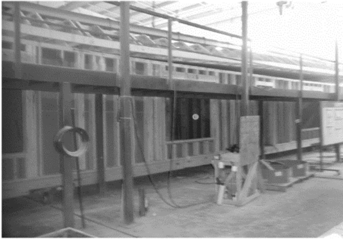
Figure 2.4.2 Permanent scaffolding erected around building modules on a Factory floor. Photo by Hopkins, Anthony Scott.
