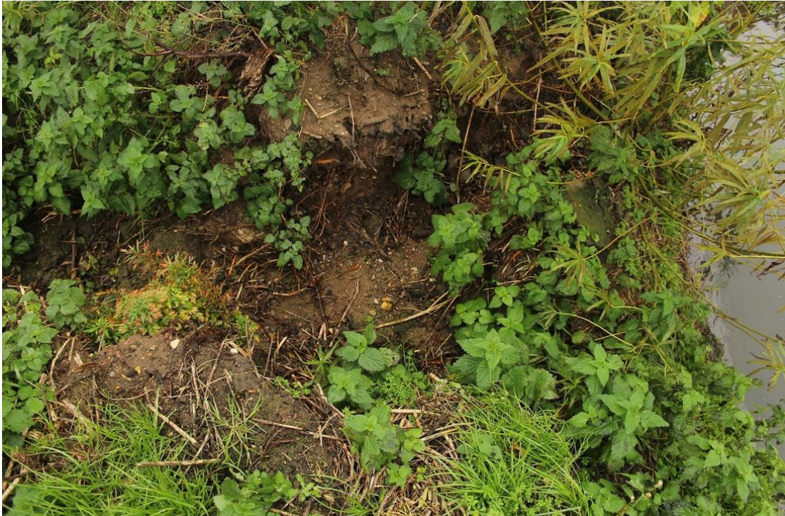
Figure I. 7. Showing of the crack in the side of basin
