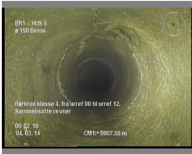
Figure I. 1. Picture from CCTV of Engvej in Hørning showing cracks in the pipe grade 4
