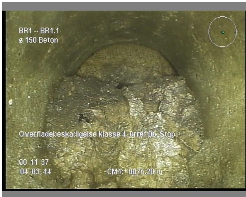
Figure I. 2. Picture from CCTV Picture from CCTV of Engvej in Hørning showing a collapse of the pipe
