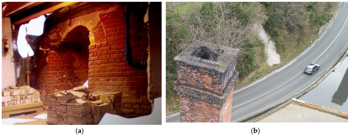
Figure 22. Captures by UAV: (a) Partial textured mesh of the entrance to the ovens on the ground floor; (b) Detail photography of the pathologies of the chimneys (Source: Authors).
