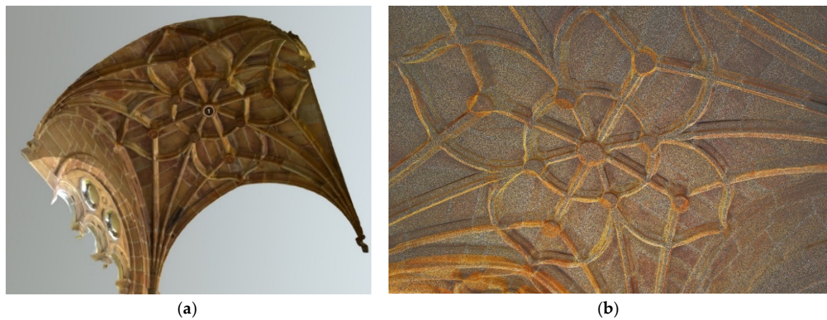
Figure 27. (a) Textured 3D partial model in Sketchfab; (b) Vault point cloud (Source: Authors).
