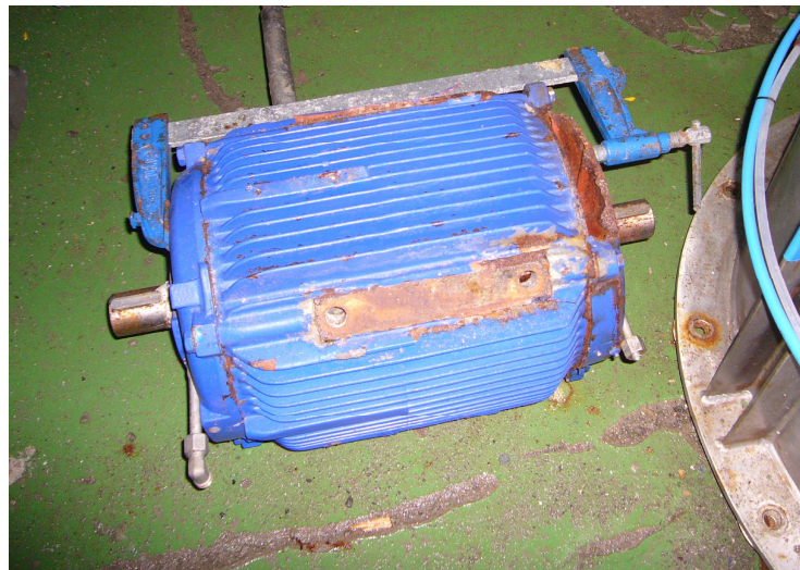
Fig. 2.37: Picture of the corrosion around a generator frame at Mutriku
