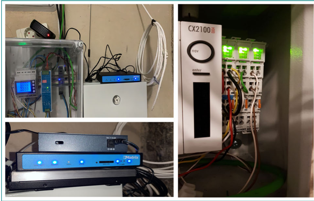
Figure D.14: Hardware and electricity meters of Mobile MCS (Co-Heating Co-Heating).
