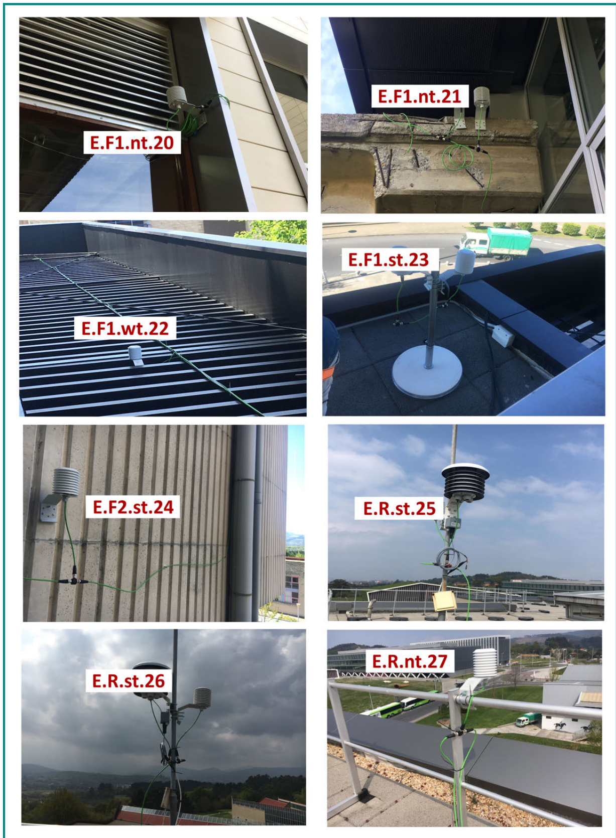
Figure A.17: Installed exterior MMS sensors' pictures [139].
