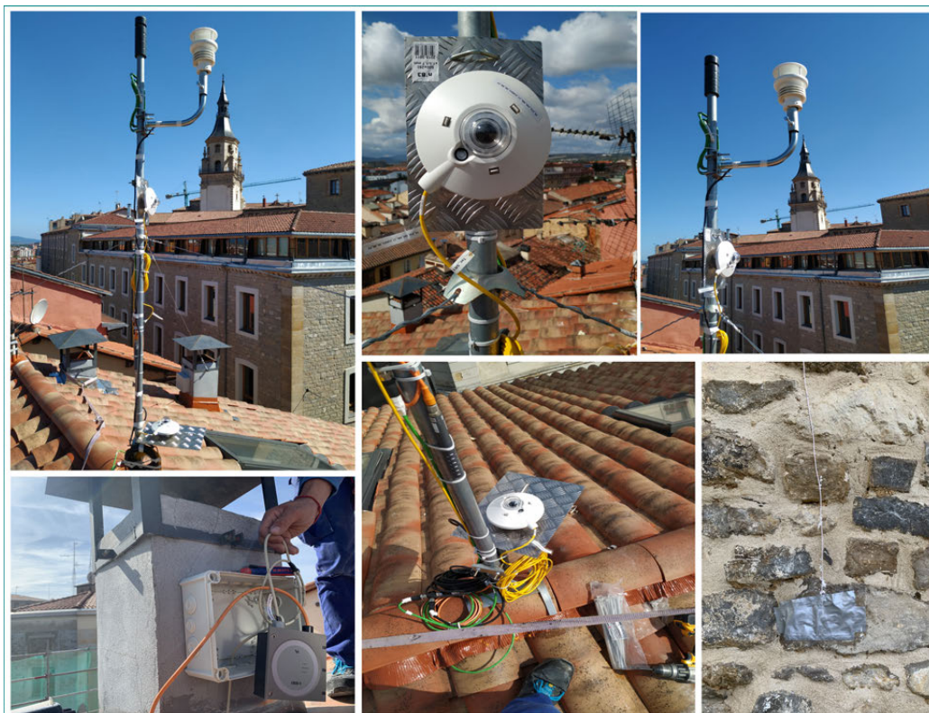
Figure D.13: Installed outdoor sensors of Fixed MCS pictures in roof.
