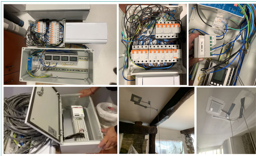
Figure D.15: Hardware and electricity meters of Mobile MCS (mobile Co-Heating).
