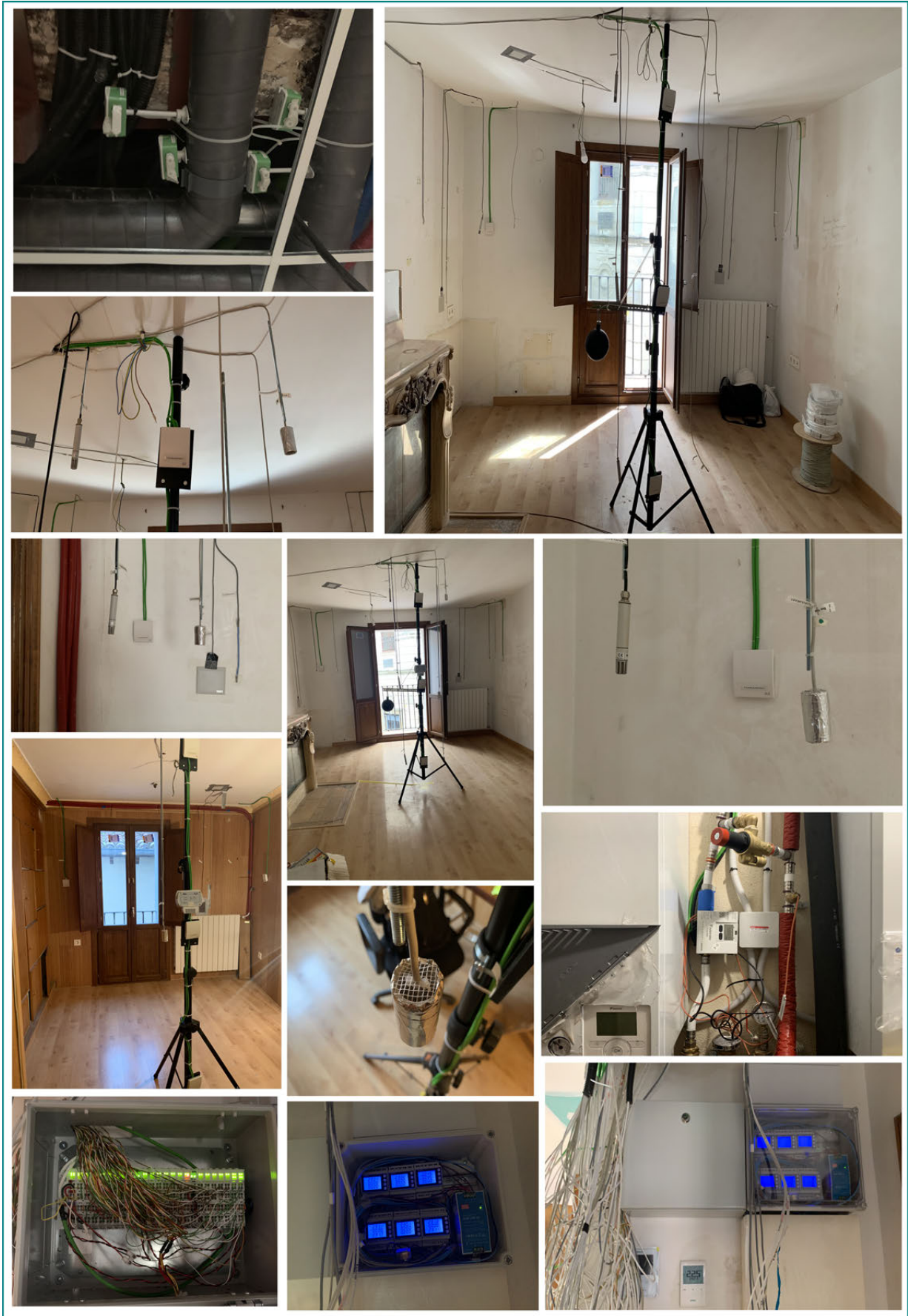
Figure D.11: Installed indoor sensors of Fixed MCS pictures in F1.
