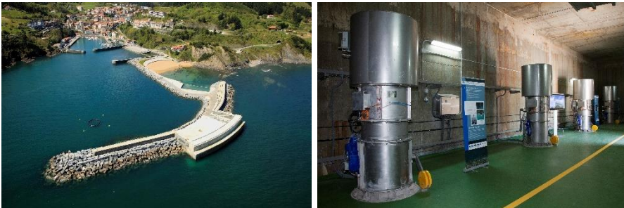
Figure 8 Breakwater in which the fixed OWC chambers are integrated (left) and some drivetrains mounted over the corresponding chambers (right). Courtesy of Ente Vasco de la Energía [36]
