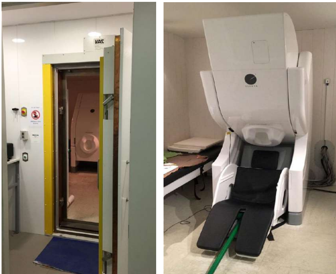
Figure 9: Magnetically shielded room and MEG facility installed at BCBL
