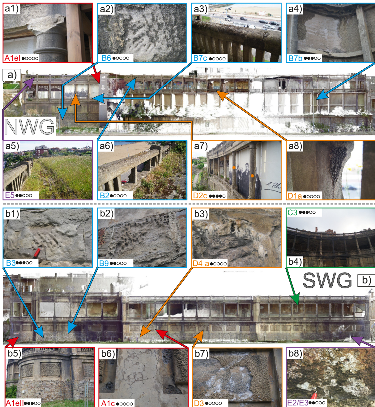
Fig. 5. Main alterations in the façades of the Punta Begoña Galleries located on the point cloud of: a) NWG (Northwest Gallery); a1) A1eI: fracture without loss of stability, breakage, of the upper part of the column; a2) B6: peeling of masonry sandstones; a3) B7c: contour flaking of plastering mortar of balustrade crosspieces; a4) B7b: spalling of decorative plaster mortar of concrete quadrants of intermediate section; a5) E5: plants on roofing; a6) B2: hiatus in balustrade crosspieces; a7) D2c: soot on façade, columns (orange circles); a8) D1a: black crusts on sides of balustrade crosspieces in the gallery corridor; and b) Southwest Gallery (SWG); b1) B3: blistering in masonry wall sandstones; b2) B9: alveolar weathering in sandstones of masonry wall; b3) D4 a: calcium carbonate encrustations in curtain walls caused by degradation of the mortar used in the masonry; b4) C3: darkening from damp area on the curved façade of the SWG; b5) A1eII: fracture with loss of stability (SWG); b6) A1c: cracking of plastering mortar of the intermediate concrete wall; b7) D3: white efflorescence on reinforced concrete of the intermediate quadrants; b8) E2/E3: bioalteration from lichen and mould. (Degree of effect: ○○○○○: no ASA; ●○○○○: <10 % ASA; ●●○○○: 10 % to 25 % of ASA; ●●●○○: 25 % to 50 % of ASA; ●●●●○: 50 % to 75 % of ASA; ●●●●●: all ASA) (based on Damas Mollá et al., 2018).
