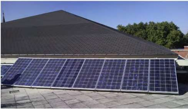
Fig. 3 e Photovoltaic modules installation (8 pieces), in University College of Engineering of Vitoria-Gasteiz (University of the Basque Country, Spain).
