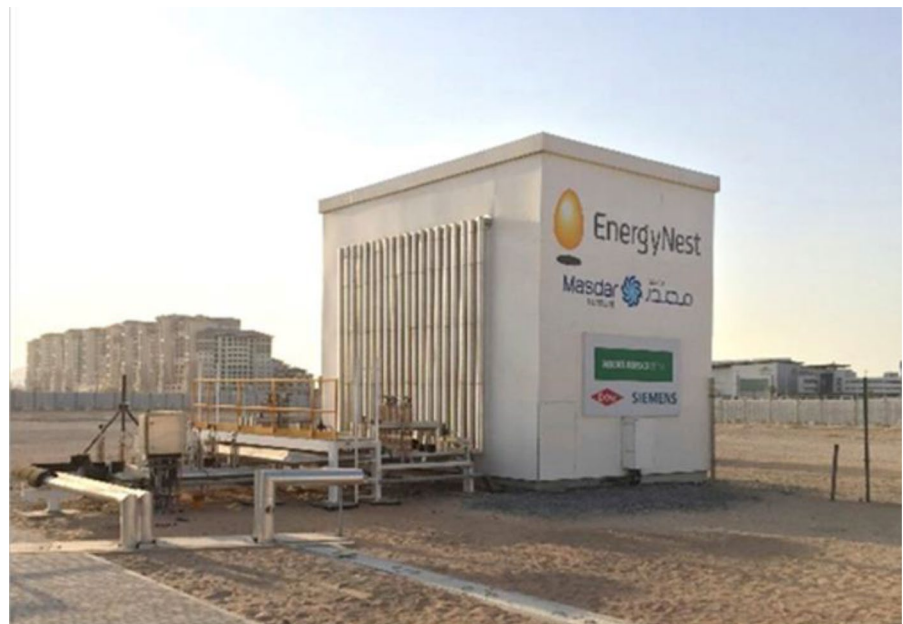
Fig. 9 Photograph of fully commissioned EnergyNest thermal energy storage with 4 × 250 kWh th capacity at Masdar Institute Solar Platform, United Arab Emirates [103]
