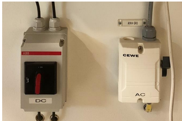
Figure 8 DC and AC switches in building 45 of the University of Gävle
