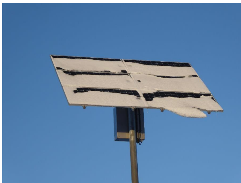
Figure 52 Solar panels covered by snow in the PV system of HiG
