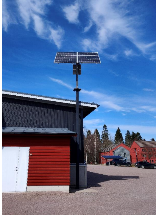
Figure 18 PV-system of building 45 in the university of Gävle
