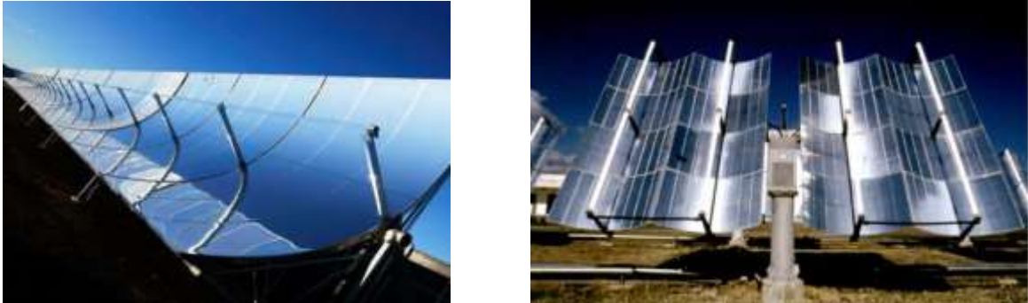
Figure 10. Collectors with one and two axes solar tracking.
