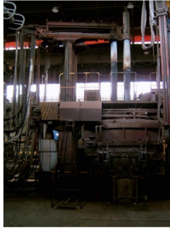
Fig. 6.4: Pilot Electric Arc Furnace (6 tones) in ArcelorMittal Global R&D center in Maizière (France).
