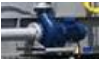
Figure 3. Condenser Spray Pump
