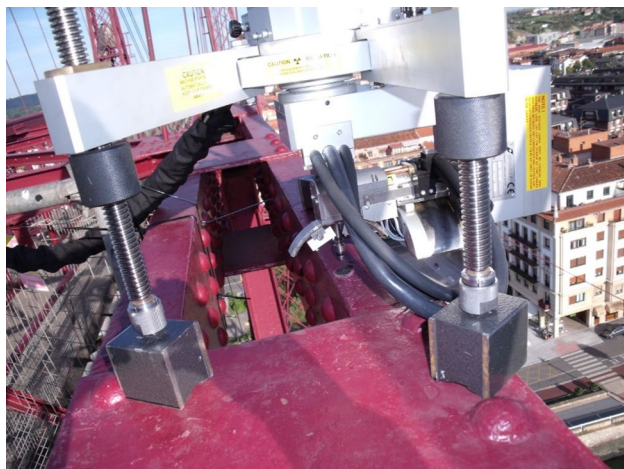
Fig. 8 Portable arrangement of the equipment on the Bizkaia Bridge at a height of 60 m
