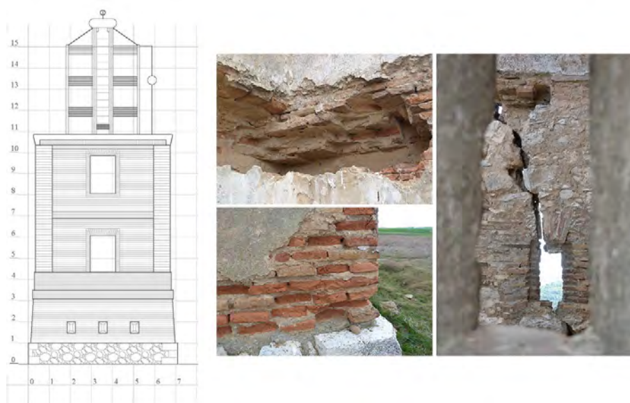
Figure 41: Façade of brick towers before whitewashing and common ailments. Left: Loss of material in Transilla. Right: Stress fractures in Tariego. (Representation and photographs by the author, 2019).
